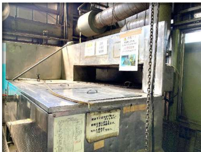
臭素系溶剤三槽式脱脂槽
